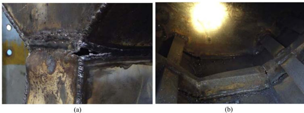
图 1 (a)支柱体与腋部连接处和(b)腋部内结构的局部断裂 [15] Fig. 1 Local fracture of (a) the connection between the strut and the haunch and (b) the inner structures in the haunch [15]
